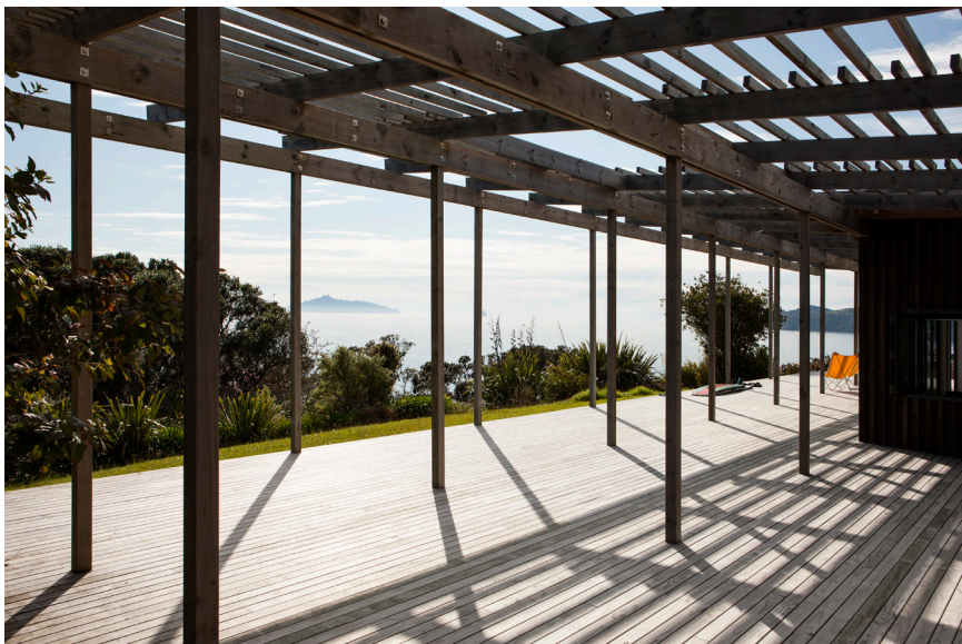
02;03;04: The old house at Langs Beach; Timber being removed and sorted during demolition; Langs Bach, Northland.
